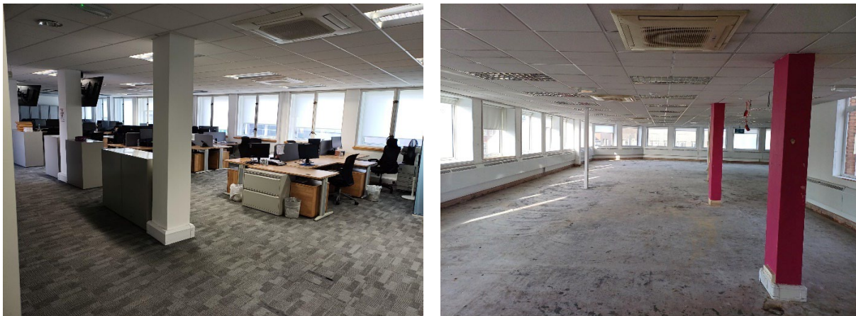
Figure 6 - Internal photographs of the existing offices at second (left) and third (right) floor level.
